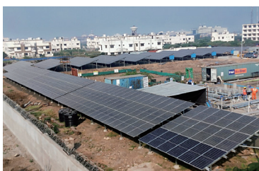
Solar power generation facilities of Gujarat Plant of Toyo Ink India Pvt. Ltd.
