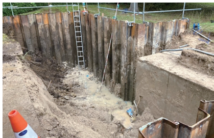
Excavation and removal of contaminated soil (Advanced Materials Research Laboratory, Toyo Ink SC Holdings Co. Ltd.)
